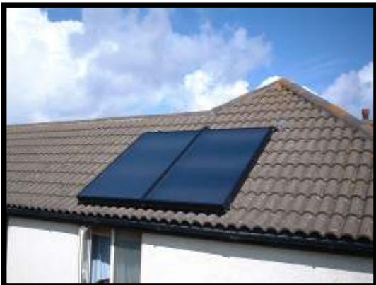
An example of a small flat plate solar hot water installation.
