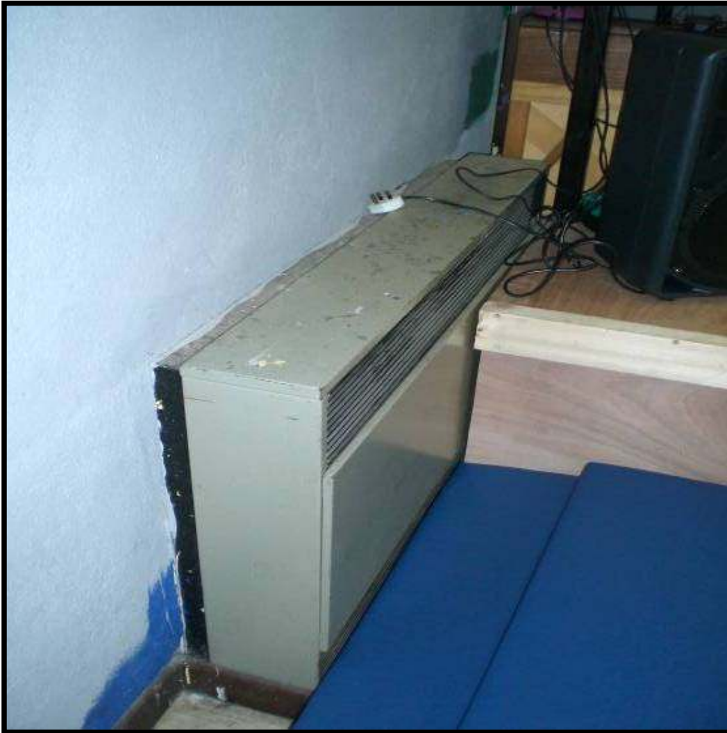
An example of the radiators in the main hall of the school.
