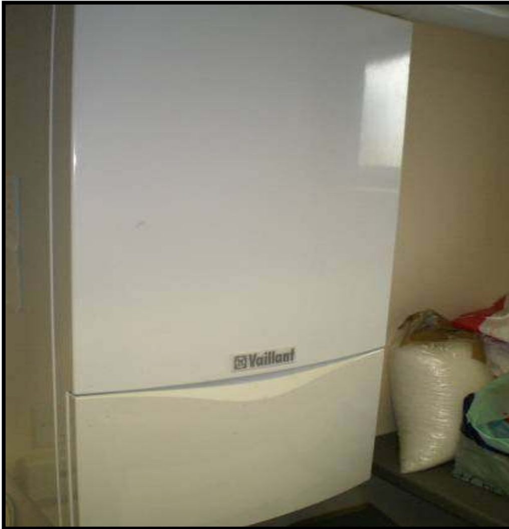
The new gas boiler in the new class rooms.
