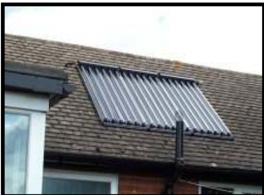
Evacuated tube solar hot water array.
